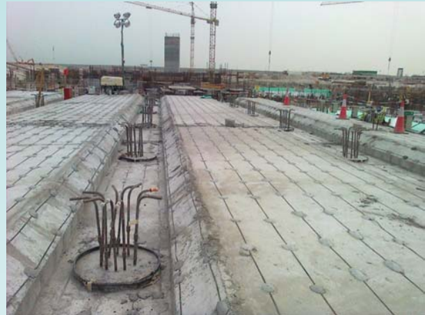
Anodes fixed to the concrete surface prior to the application of a second layer of screed
