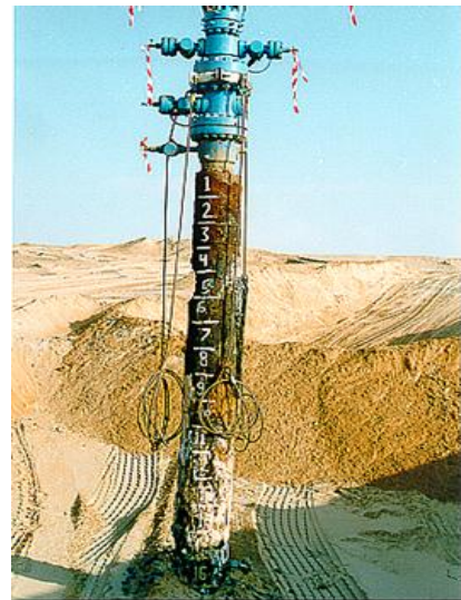
Surface Corrosion of Well Casing
